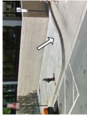
Missing Curb Ramps
