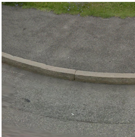
missing curb ramp
